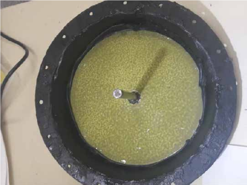
Fig. 8.- Diaphragm assembly stuck to the casing
